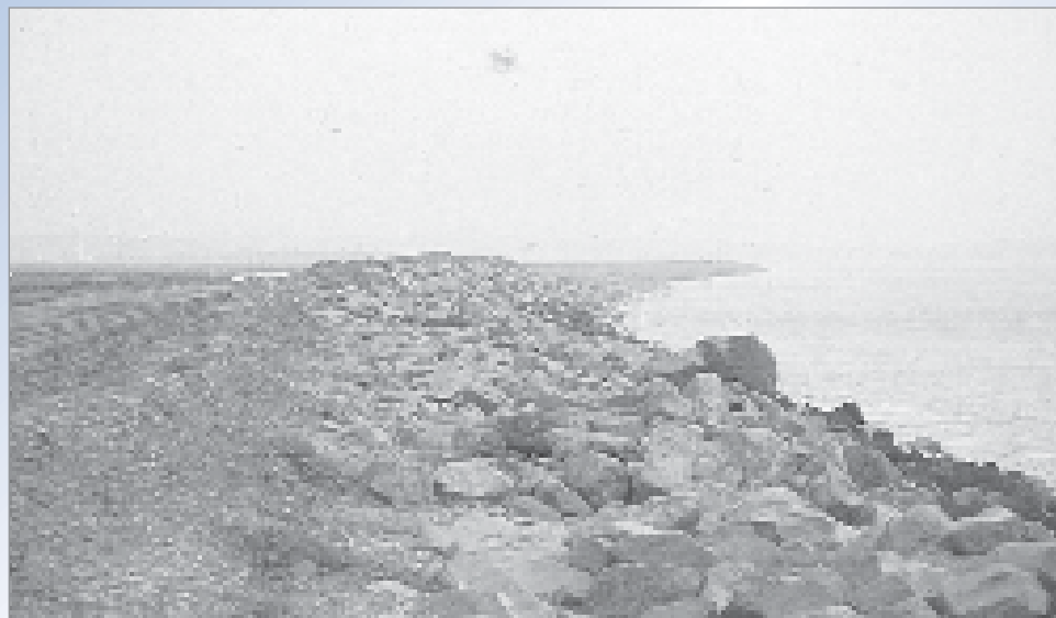
Figure 10.9 Hurst Spit armourstone revetment in December 1989, after storm damage (courtesy A P Bradbury)
