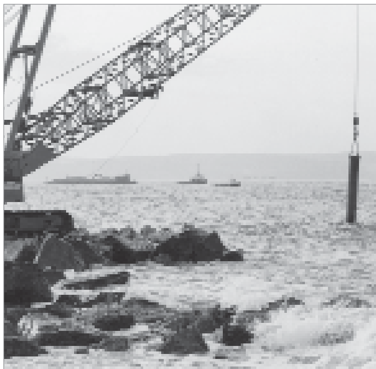
Figure 10.12 Profiling the submerged section of a breakwater by soundings from a crane (courtesy David Bowie Photographic)
