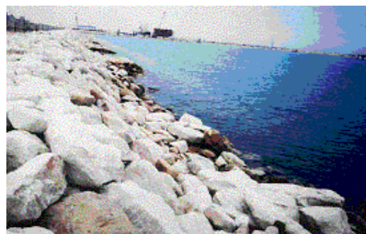
Fig 16: sinusoidal damage of Berm edge
