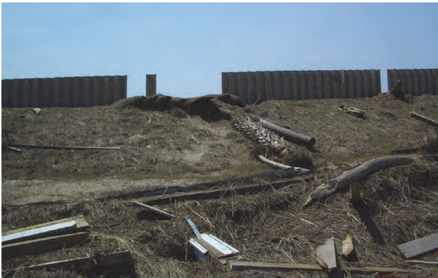
Figure 3.25: Debris such as logs in the water broke a pvc sheetpile during a hurricane and the material was transported over the crest to the landward slope. Picture taken from inside, looking at the landward slope. Gulf coast, USA
