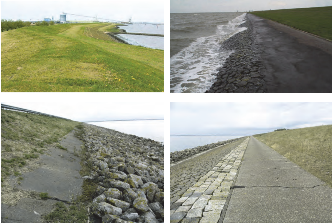
Figure 5.1: Examples of coastal dikes, levees and seawalls. Delfzijl, NL; Busum, DE; Houtribdijk, NL; Rotterdamse Hoek, NL
