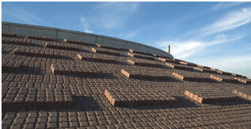
Figure 5.32: Rib pattern produced with two thicknesses of place block revetments. Each area of 4 by 5 units is placed mechanically in one move. Courtesy Projectbureau Zeeweringen
