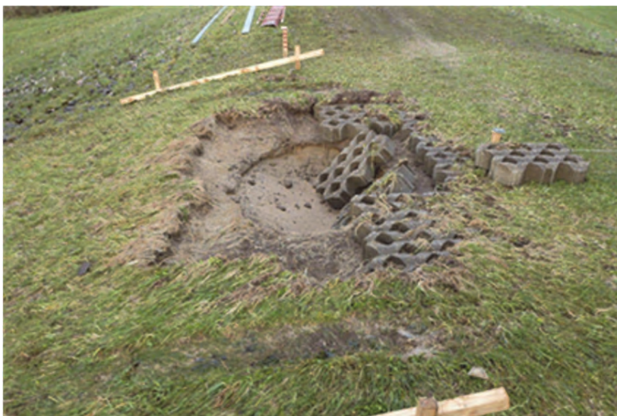
Figure 4.43 Failed road crossing by under-mining due to simulated wave impacts
