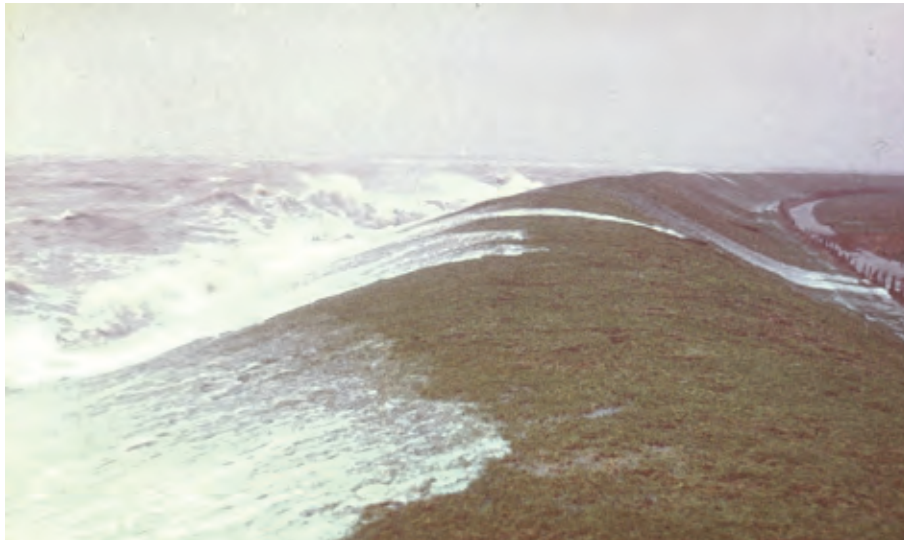
Figure 5.34: Short-crested waves resulting in wave run-up and wave overtopping (photo: Zitscher)
