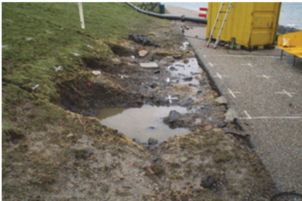
Figure 4.39 Final damage after the pilot run-up test
