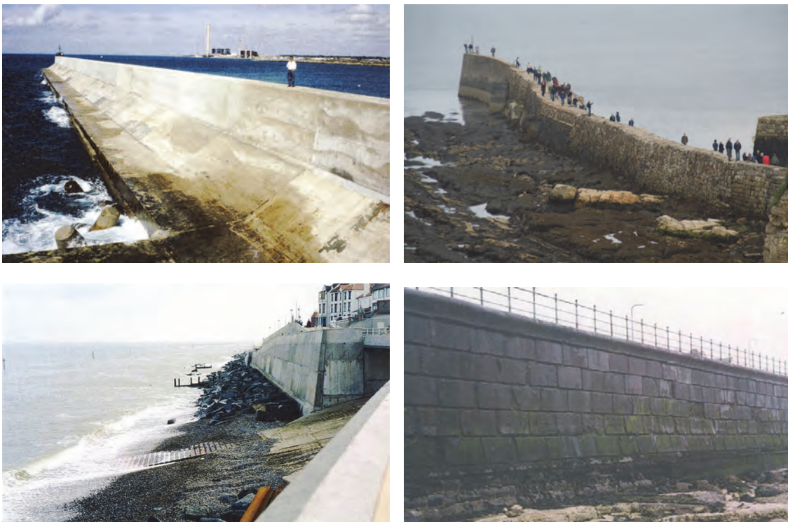
Figure 7.1: Vertical structures: (clockwise top left) modern caisson breakwater with shifted parapet (Civitavecchia, Italy), old blockwork breakwater (St Andrews, UK), modern concrete seawall and older stone blockwork seawall with bull nose
