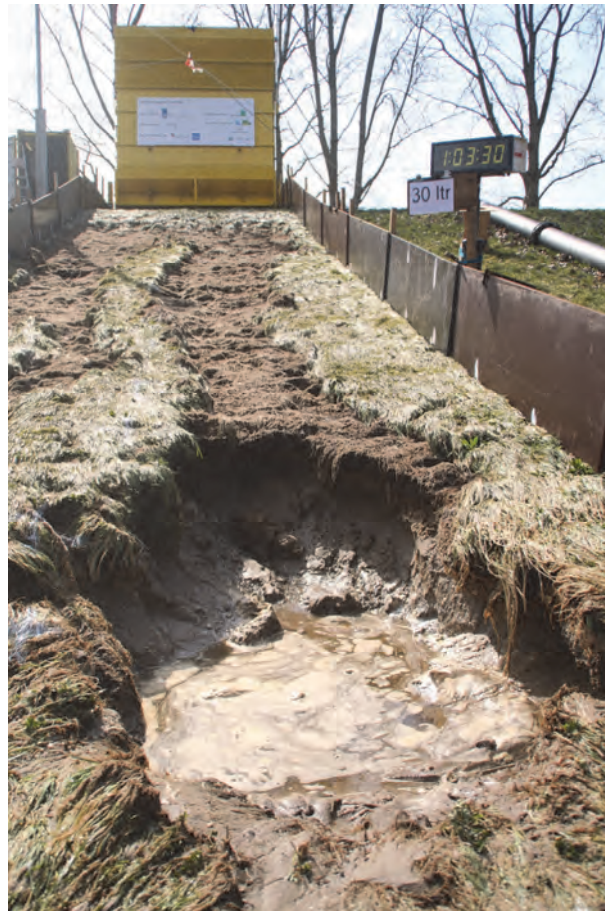
Figure 4.35 Failure of a grass covered sand dike
